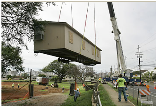
DENNIS ODA / DODA@STARBULLETIN.COM Hawaii Modular Space delivered modular buildings yesterday to temporarily replace a UH Lab School building that was destroyed by fire.
